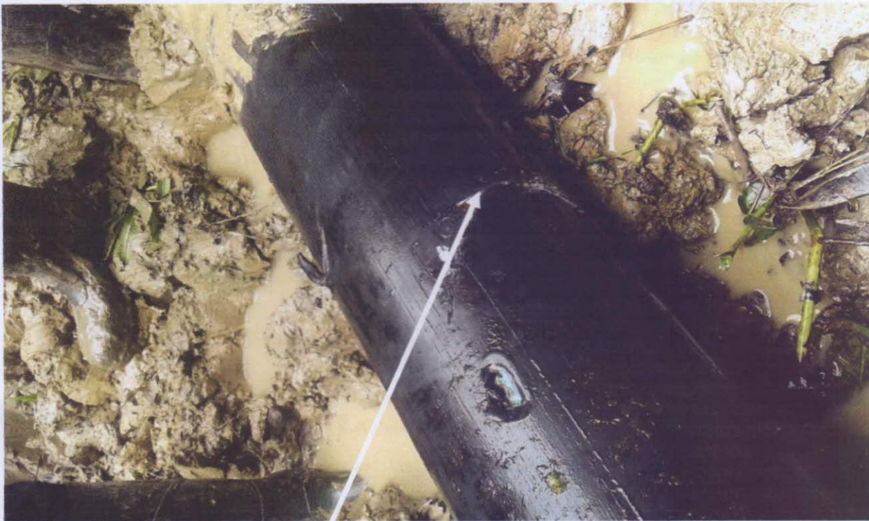
LEAK POINT (HACJ. SAW CUT WITH EFFECTIVE OF 110MM)
